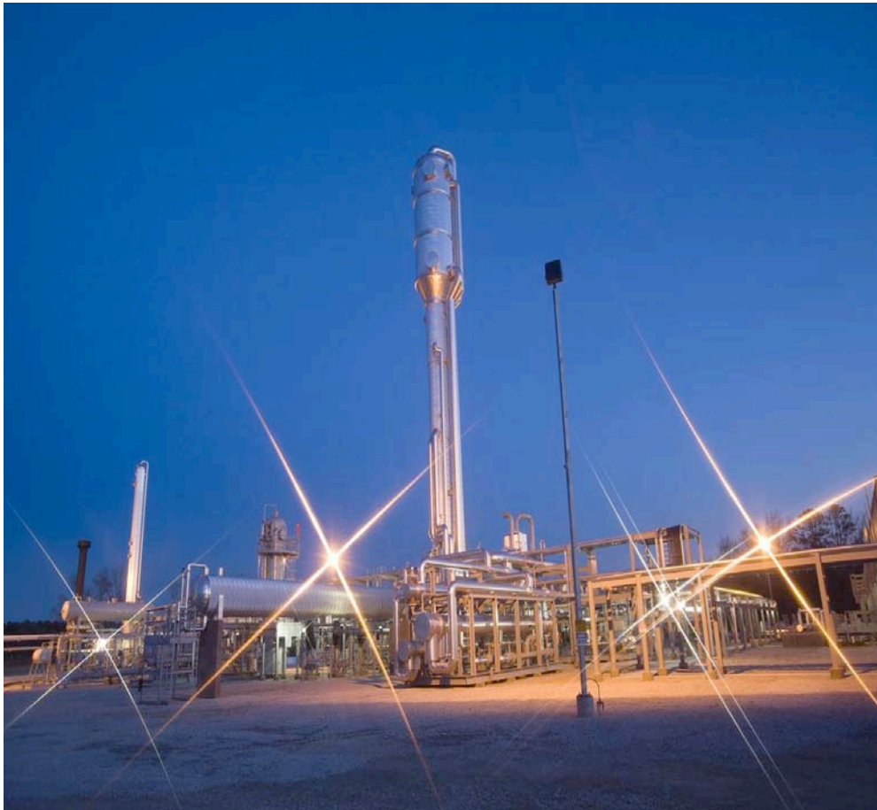
Figure 14: Natural Gas Processing Facility
